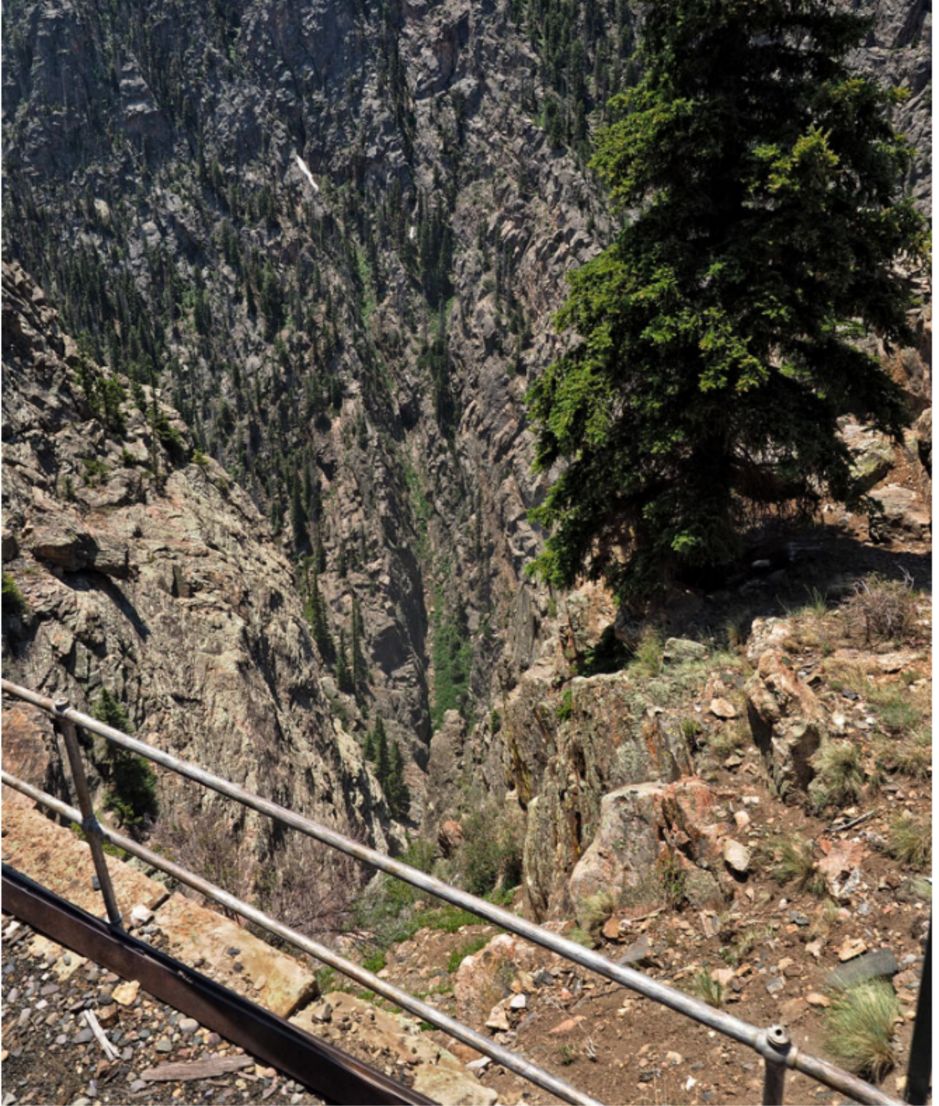
This is the view as the train pops out of the tunnel. You can barely see the river far below the track.
